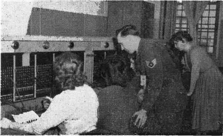
French Civilian telephone operators at the Base Comm Center repeat the familiar phrase, "Number, please", approximately 5,000 times daily. Pictured above, observing the day shift at work, are: S/Sgt Lyndell L. Mundy, Switchboard NCOIC and Jacqueline Binsinger, Civilian Supervisor. (Complete story on page 2.)
