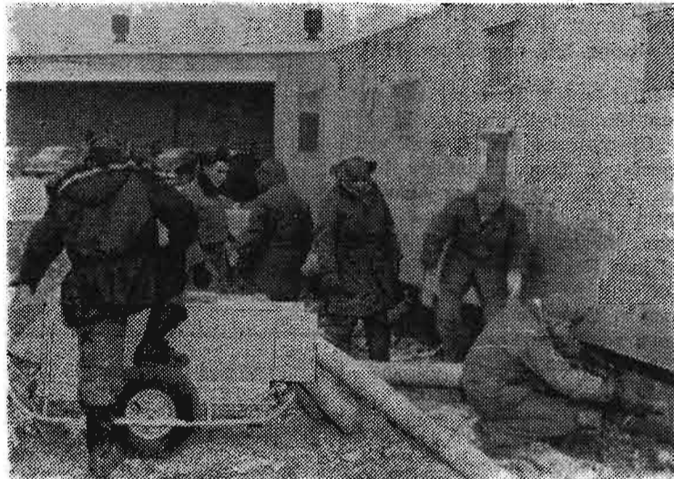
Personnel of the 416th Fighter Bomber Squadron, pictured above, worked under extremely adverse weather conditions last week while thawing out frozen water pipes in the Chambley Base Trailer Park. Pictured from left to right are S/Sgt Winford K. Moore, A/1C Paul F. Slatniski, A/2C James H. Cox, S/Sgt Arthur R. Noriega, M/Sgt John Boldt, and M/Sgt Dewey F. Savell.
